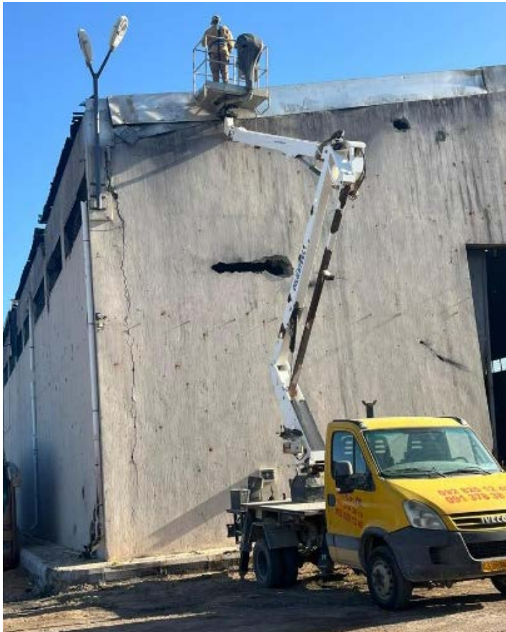
LPO EOD team removing items from elevated warehouse structures at the General Company of Ports
